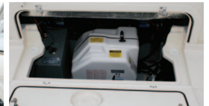
Easy access for standard generator
