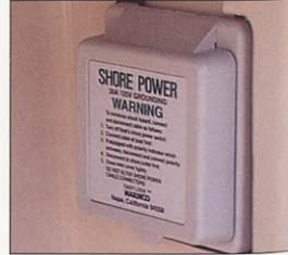
▲ Dockside power (part of a convenience package)
