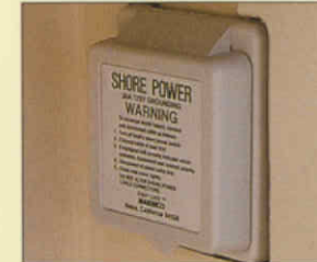
▲ Dockside power (part of a convenience package)
