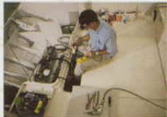
A Grady-White systems engineer performs a check at a critical stage in the installation of a Marlin 300 system.
