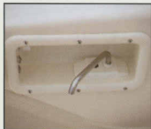
▲ Gunwale mounted freshwater system
