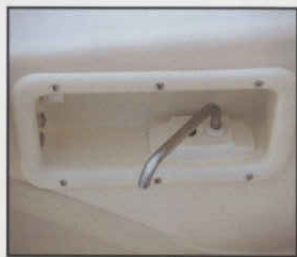
▲ Gunwale mounted freshwater system
