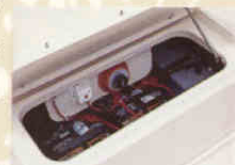
Typical pre-rigged electrical and fuel system installation.
