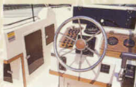
Helm area with lockable electronics box
